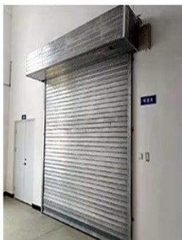
Fire shutter doors
